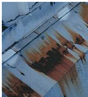
Rust and corrosion.
